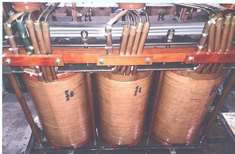
Figure 19: The other side of the transformer active part for inspection
