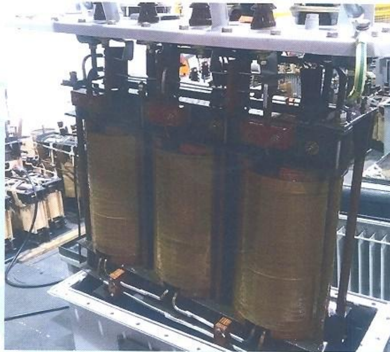
Figure 18: One side of the transformer active part for inspection
